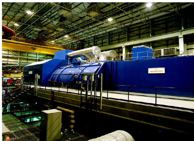
Figure 1: A steam turbine generator unit
